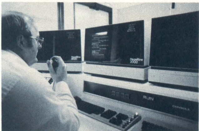
Closeup of control room console and CRT terminals. "Field" operators communicate via 2-way radio with process operator who interfaces with computer
